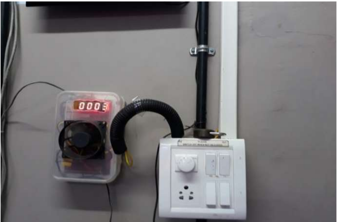
Image 3 – Room automation console
